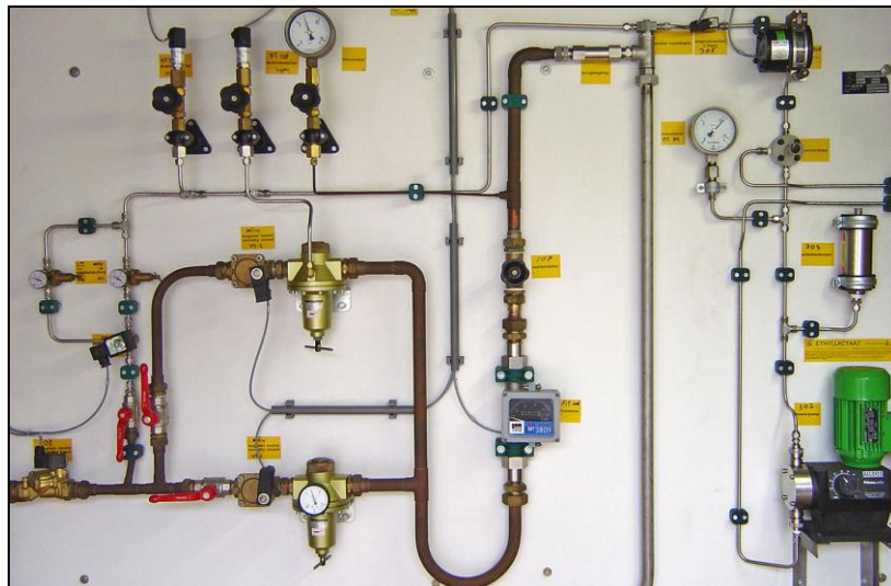
FIGURE 2.28. INJECTION SYSTEM CONTROL PANEL.
