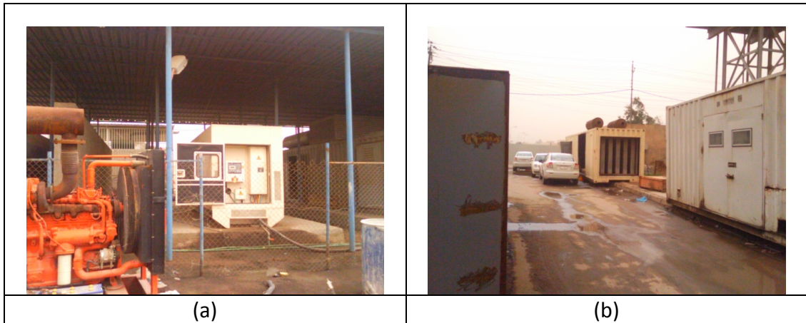
Figure 5.11: Standby generation facilities in (a) Basra General Hospital (within the fence) and (b) three unused units.
