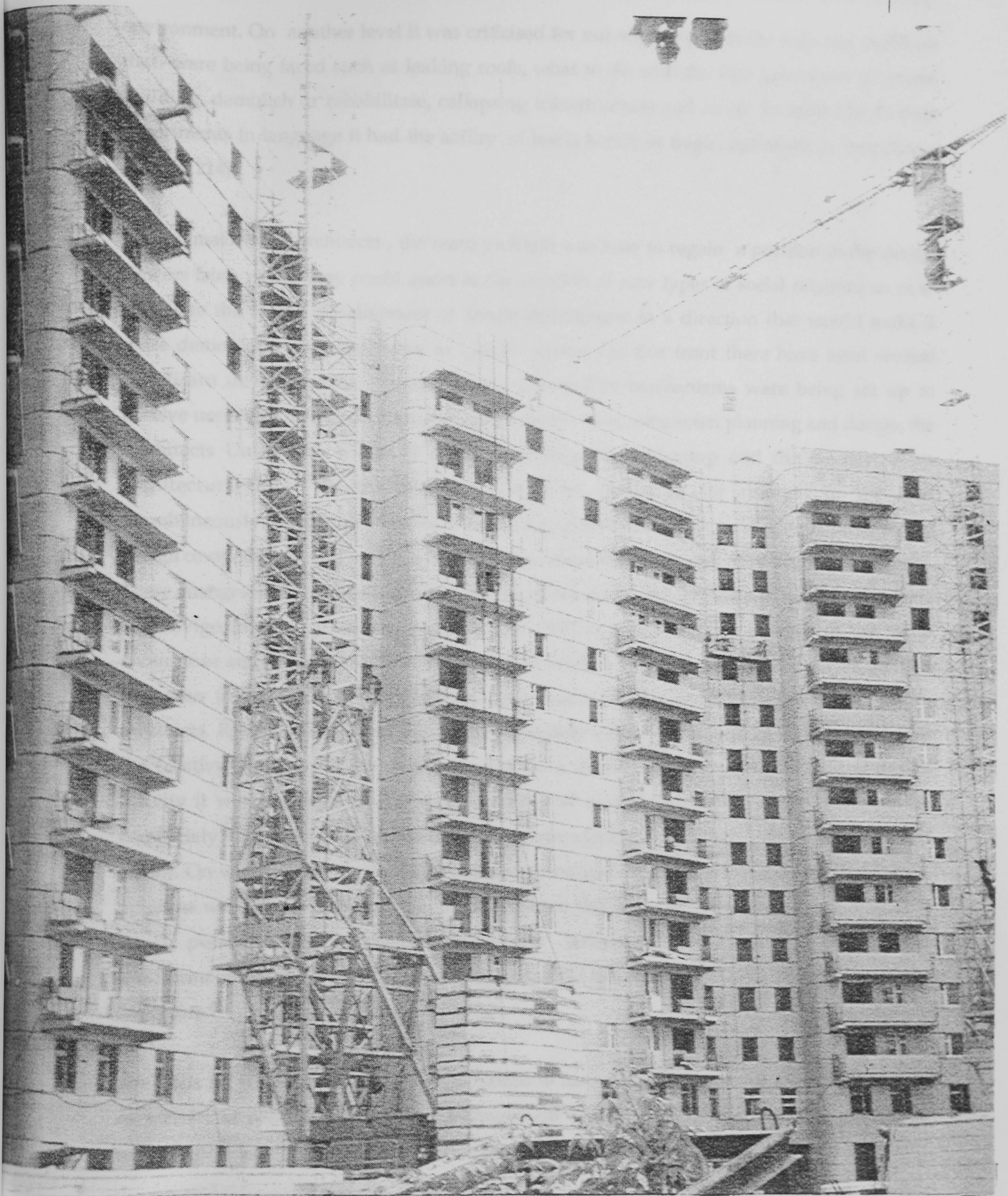
The attempt to introduce a greater flexibility and diversity into the mass pre-fabricated production of concrete panels and components. Moscow, 1988
