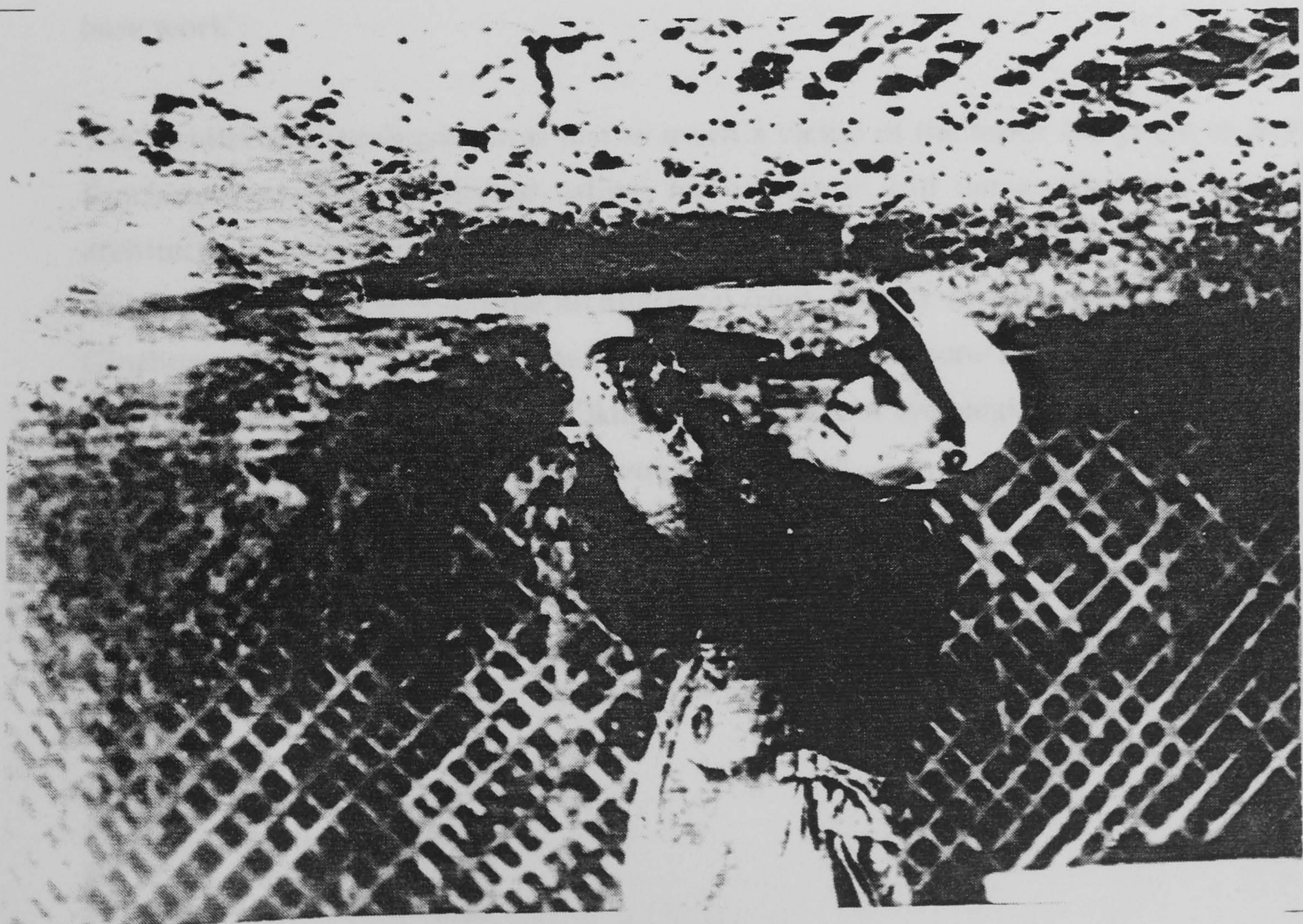
Plastering over the cracks, 1930's
