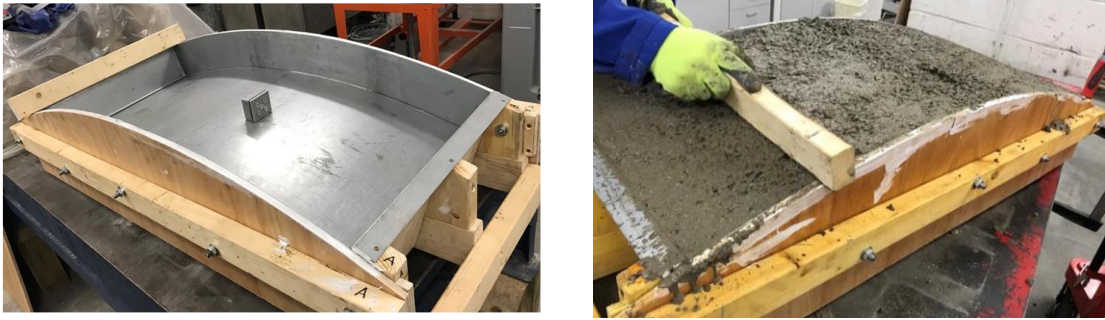
Figure 5-6. On the left the segment formwork is shown. The right shows the segment being casted.
