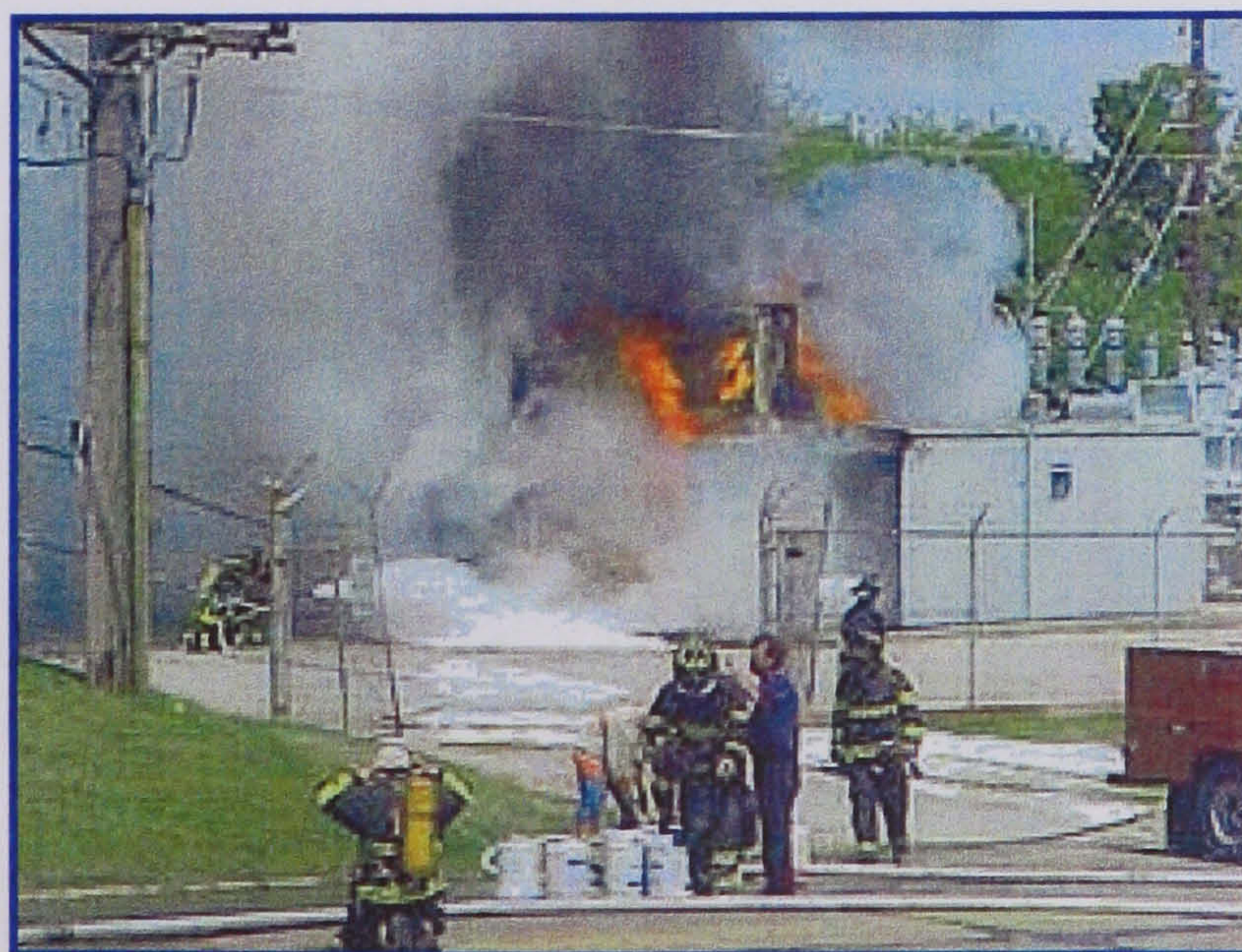
Figure 1.2 Example of a catastrophic transformer failure (photograph courtesy of Lee Lane).
