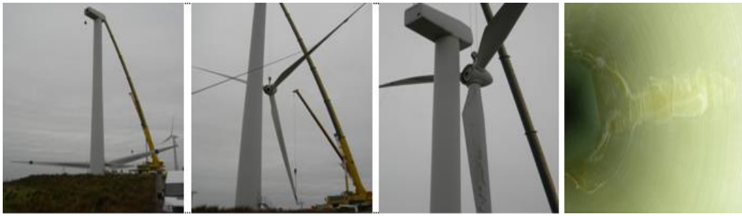
Figure 3.7: Crane support as rotor hub is lifted into position; internal blade damage & repair (right)
