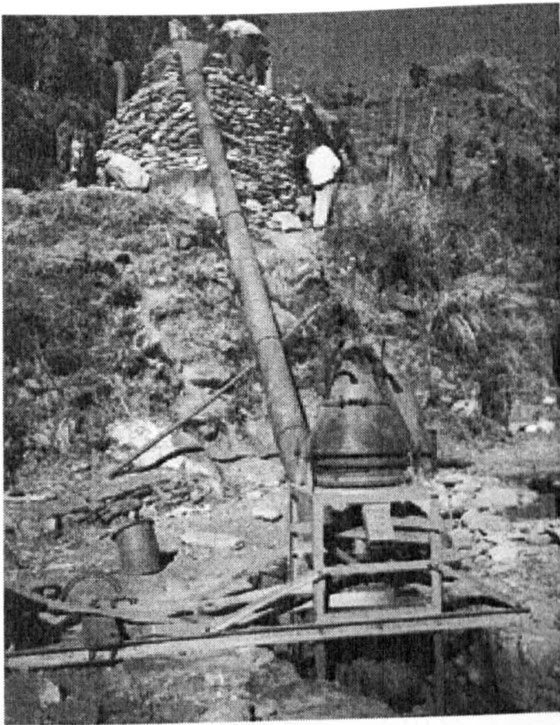
MPPU with Penstock Pipe
