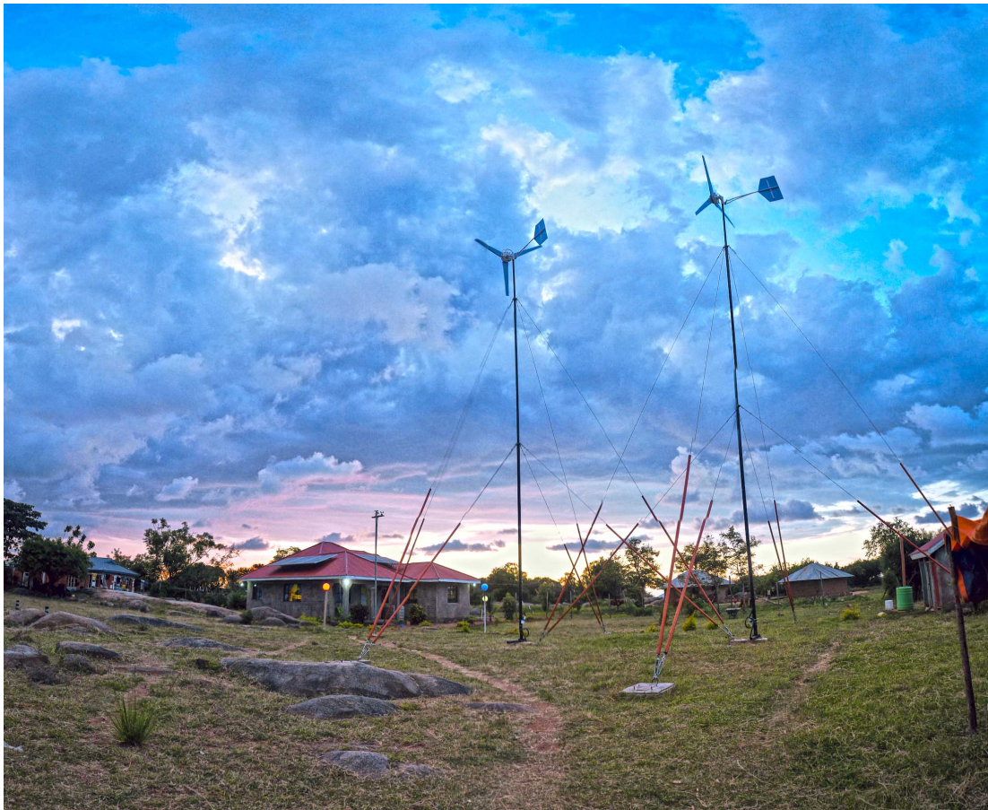
Figure 3.11: Muhuru Bay Micro Grid Turbines and Solar Panels
