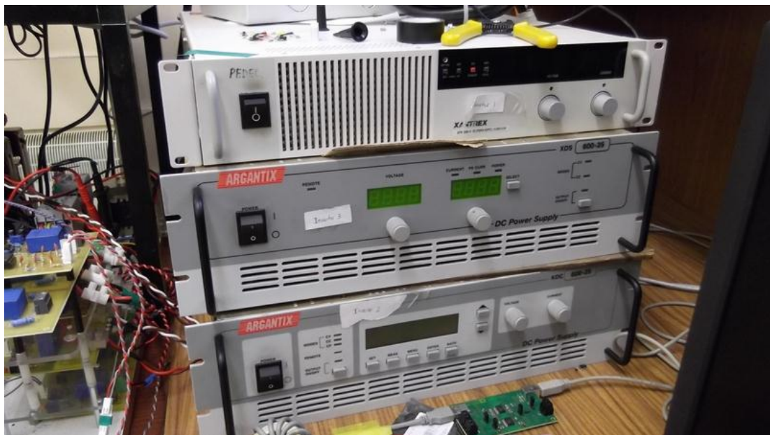
Figure A.7 Dc power supplies
