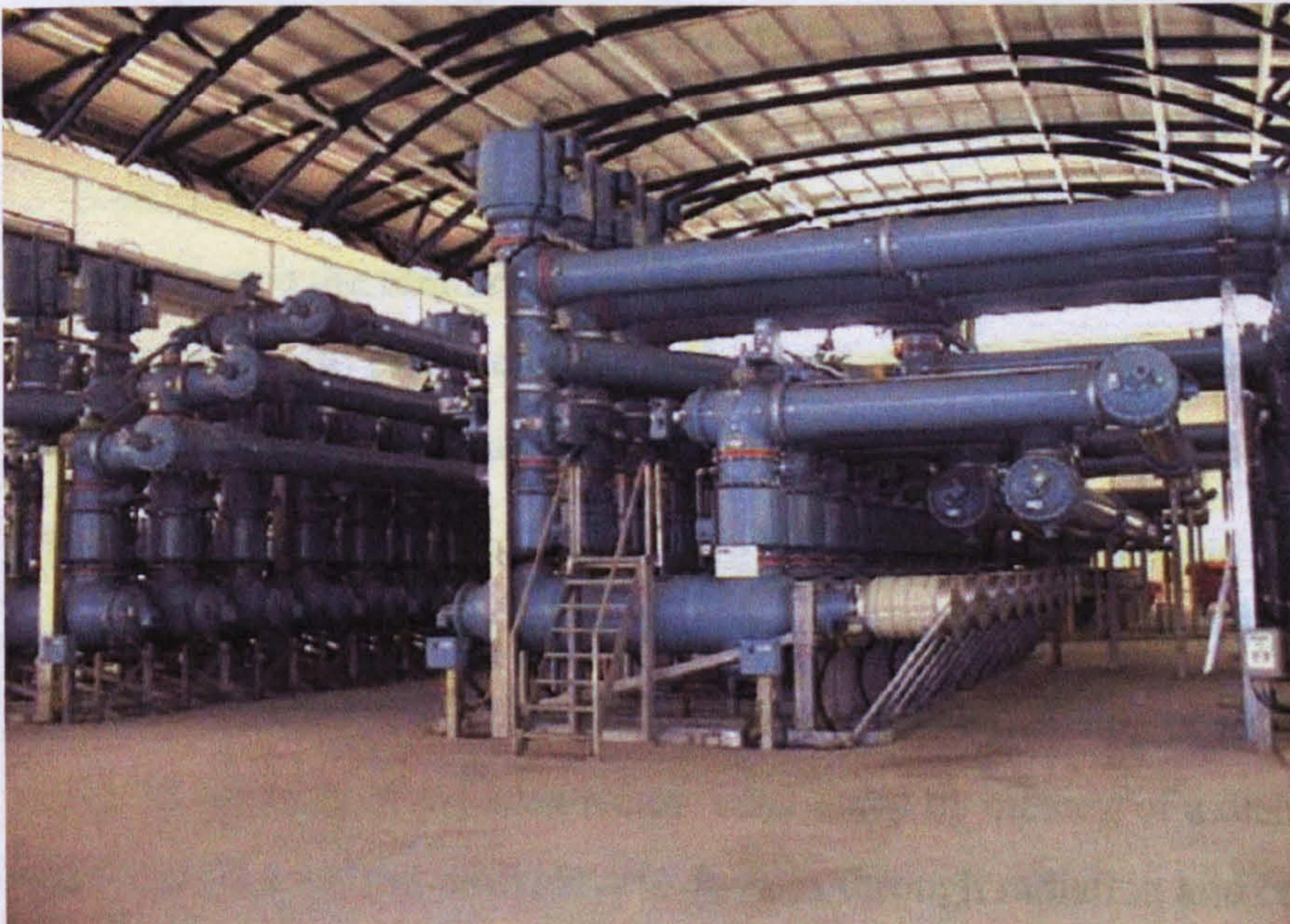
Fig. 2.2: Installation view of the gas insulated switchgears in a GIS
