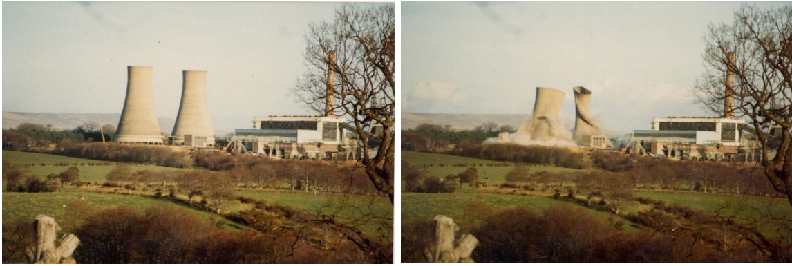
Figure 5.4: Barony Power Station on the day it was demolished in 1982. Images from ayrshirehistory.com (Tannock, 1982).
