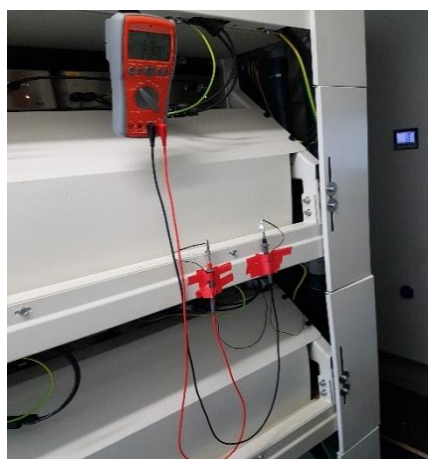
Figure 8.2 multimeter connected to single stack within the RFB
