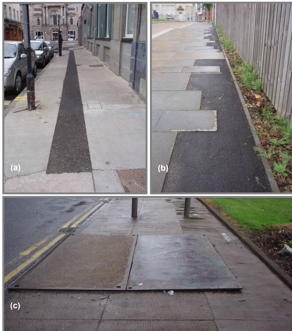
Figure 6.5: Poor pavement reinstatement (a) Garth St, (b) Shuttle St, (c) Cathedral St
