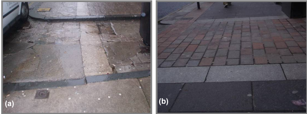
Figure 6.14: Treatment of level changes at vehicular access entrances (a) North Fredrick St, (b) Ingram St
