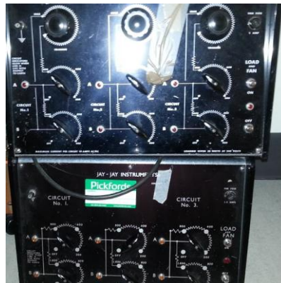
Figure A. 12. Three-phase auto-transformer
