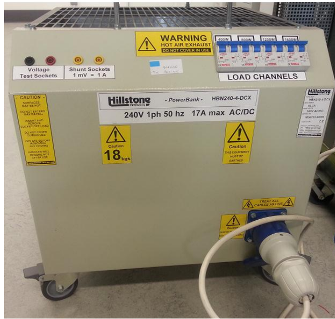
Figure A. 13. Three-phase auto-transformer
