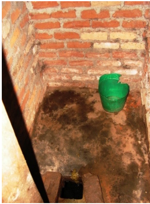
Ph. 2.10 Soiled pit latrine with no cover, Southern Malawi (May 2007)
