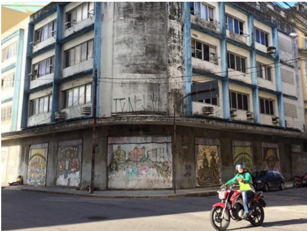
Fig. 4. Building awaiting refurbishment in port area of Recife, Brazil, (Horgan, 2016).
