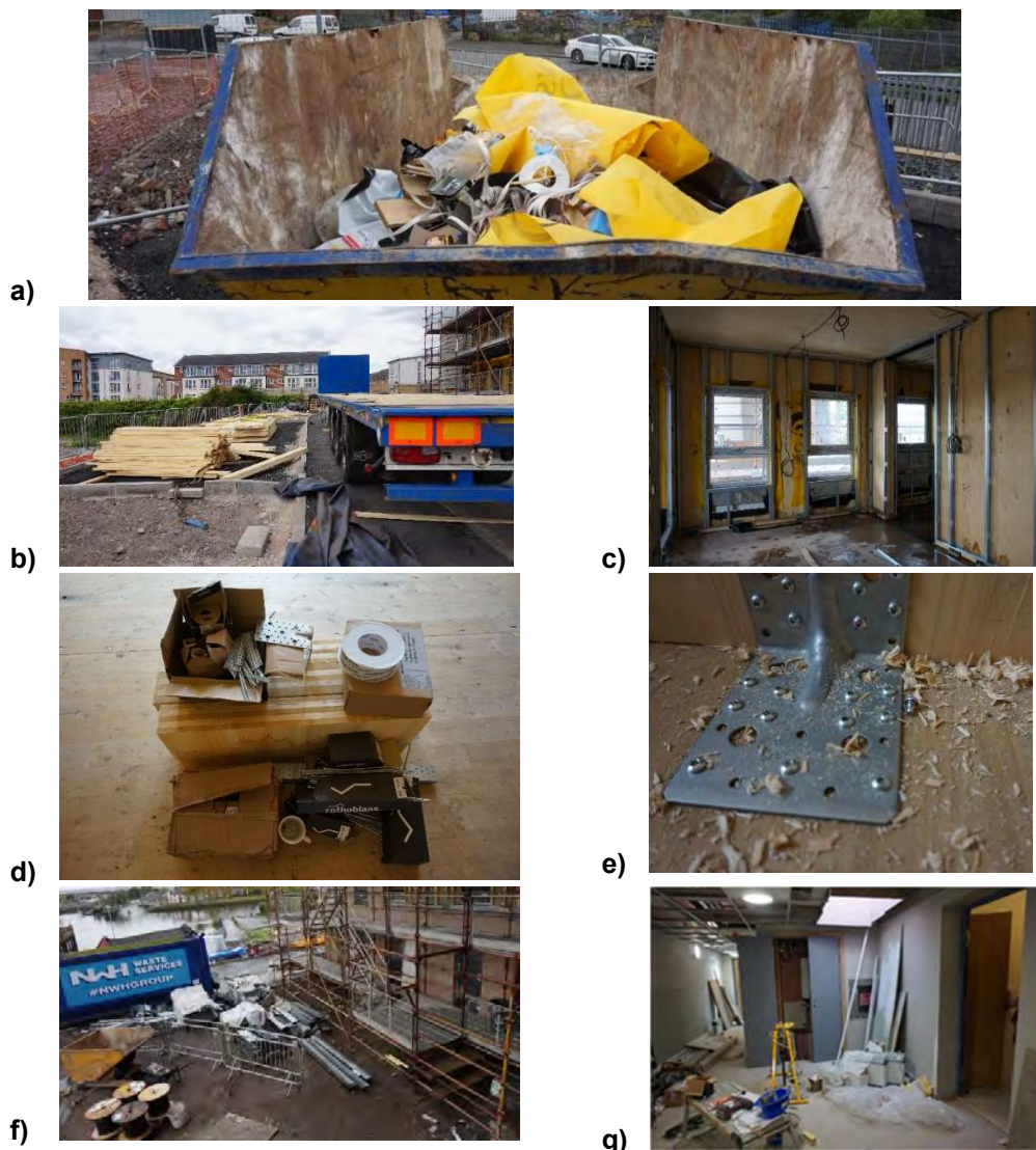
Figure 7B11. Waste observations. a) CLT installation waste; b) CLT panels stacked; c) clean internal environment; d) CLT waste; e) CLT woodchips; f) external works and g) internal works waste observations.
