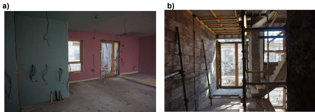
Figure 7B14. CTP case study internal works: a) CTP apartments, and b) blockwork common areas
