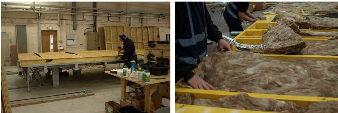
Figure 63. Examples of manual production activities, bespoke panels assembly with a manual nail gun and installation of insulation.
