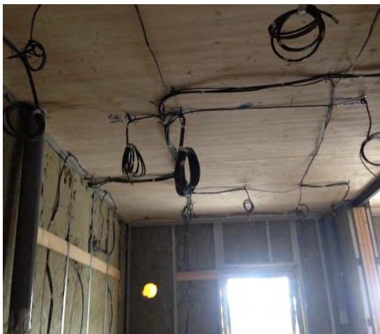
Figure 7B6. Electrical services installation at CLT case study. 30/06/17.
