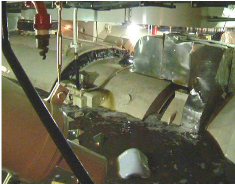
Figure 1.7. Flooding into engine room (Bole, 2007)
