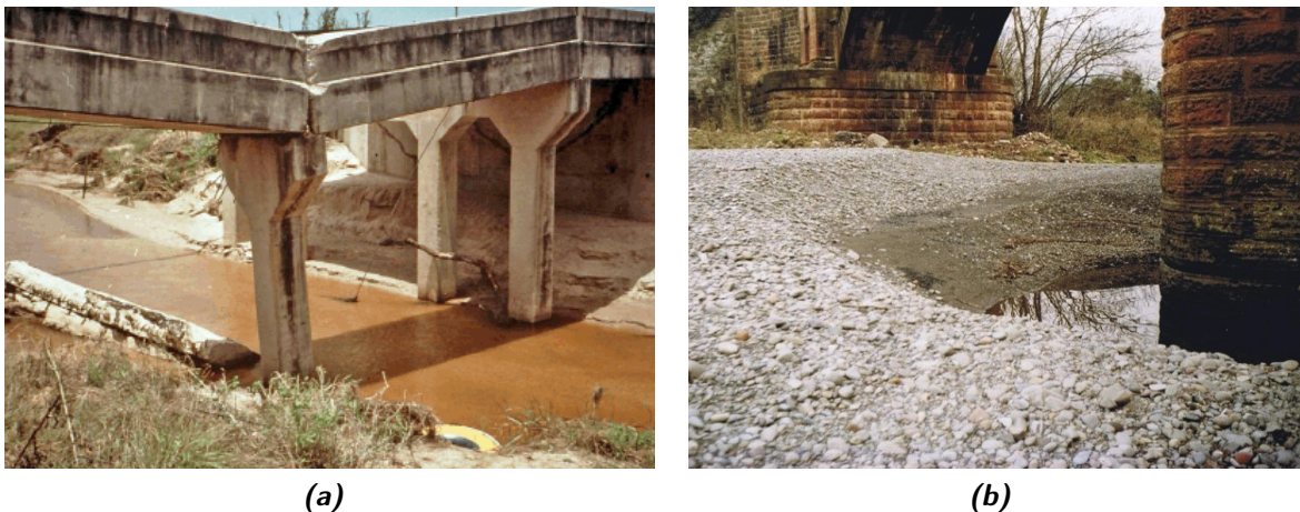
Figure 2.2: (a) Bridge failure due to scour (Texas A&M Transportation Institute, 2014) and (b) detail of scour hole around a bridge pier (Dundee Tunnel Research, 2012)
