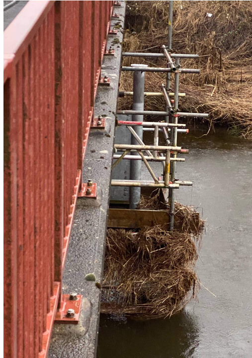
Figure 3.26: Hay and debris on the probe P_2
