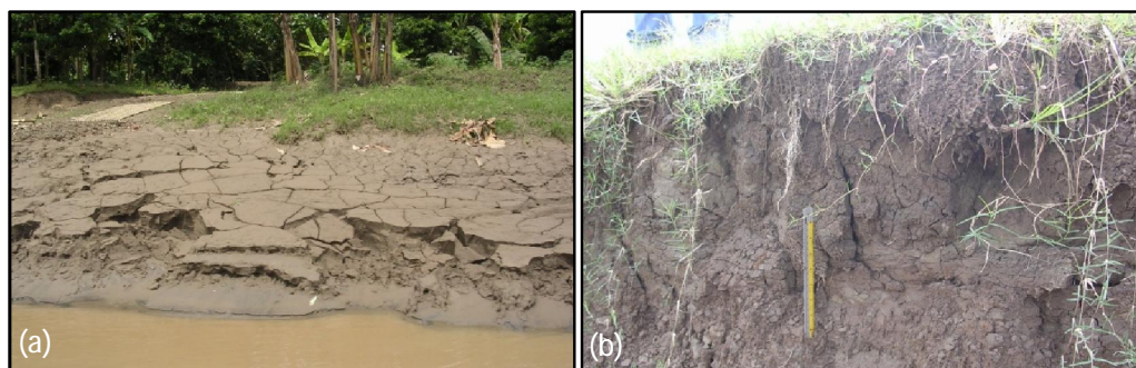
Figure 2.8: Evidence of desiccation cracks (a) on embankment face and (b) extending into embankment
