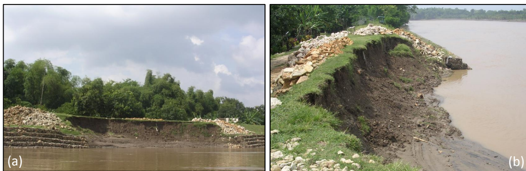
Figure 2.11: Global failure of gabion reinforced embankment (a) front view, (b) side view
