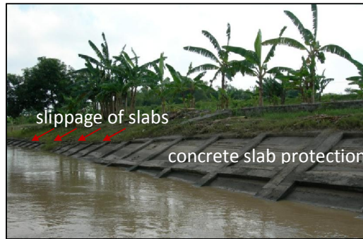
Figure 2.7: Differential settlements due to concrete slab protection
