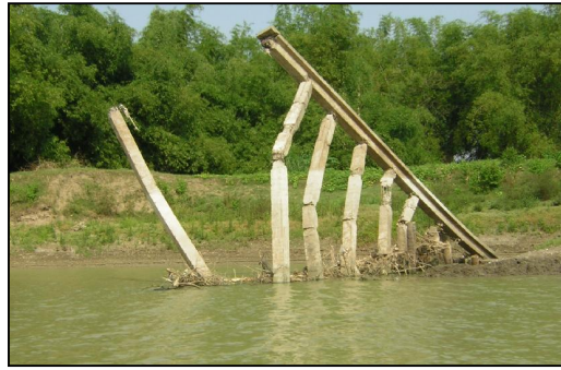
Figure 2.6: Damage of flow control structures
