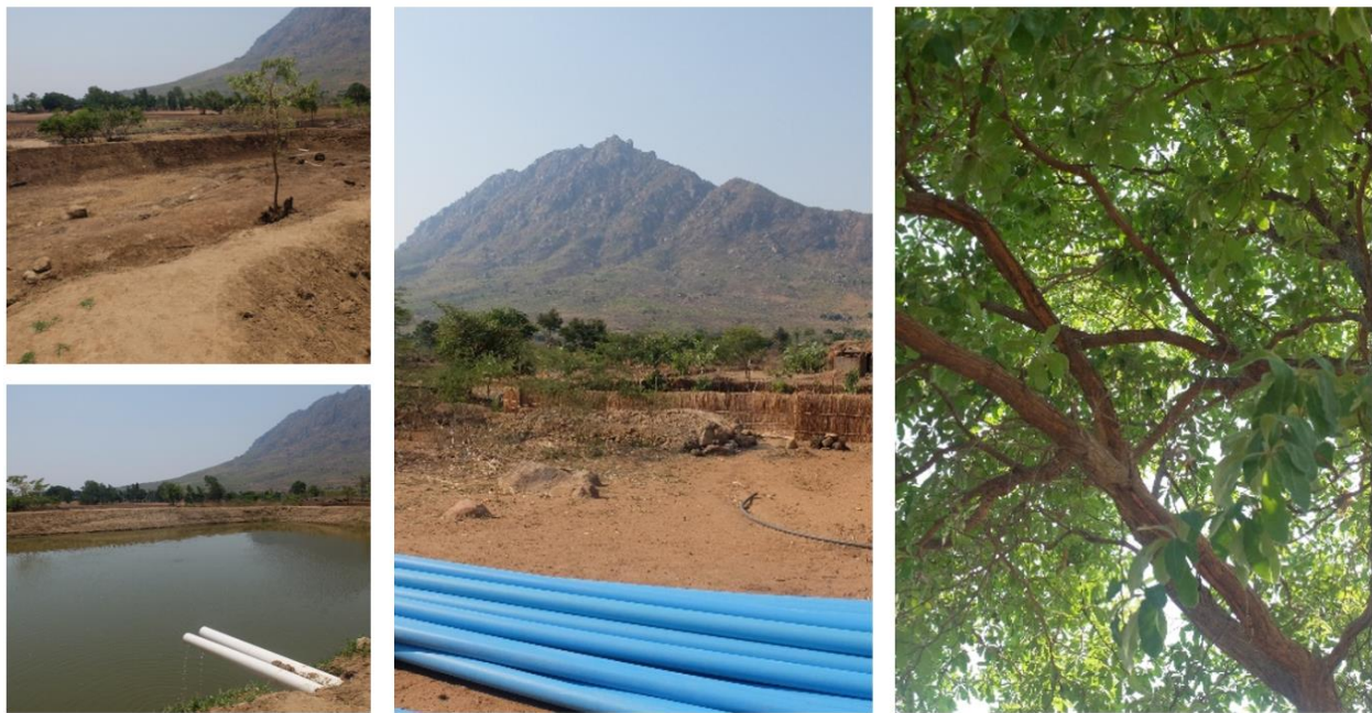
Figure 5.58: Jordan village. Images: top left and bottom left — aquaculture pond in process of construction, completed pond; centre — new pipes delivered for construction project; right — village tree under which our meeting took place.
