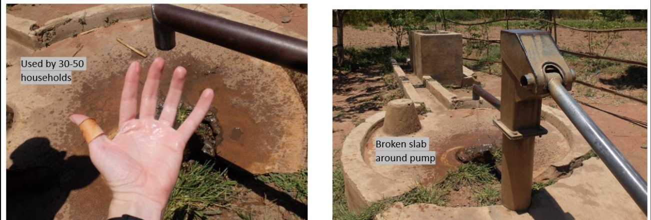
Figure 5.50: Handpump at a waterpoint, with degraded infrastructure.
