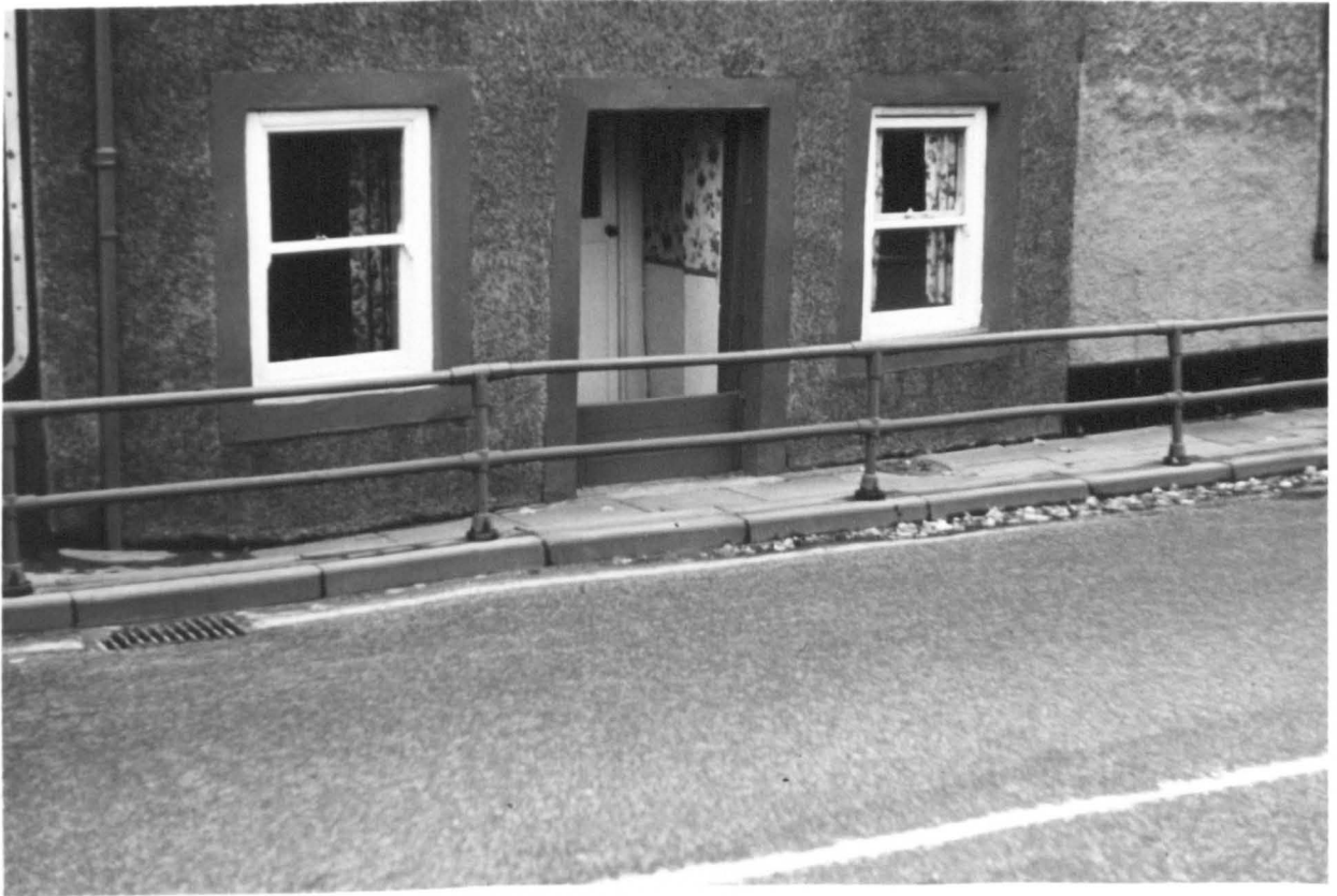
Plate 22. Appleby: The permanent flood proofing measure employed by an Appleby resident. This board has been cemented into place to prevent flood water entering the property.
