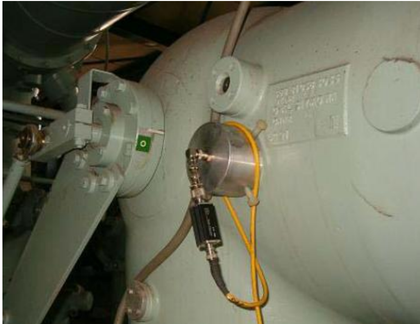
Figure 3.4: External UHF PD mounted on the inspection window of GIS tank. The sensor is connected to an amplifier with a passband between 300 MHz and 2 GHz [83].
