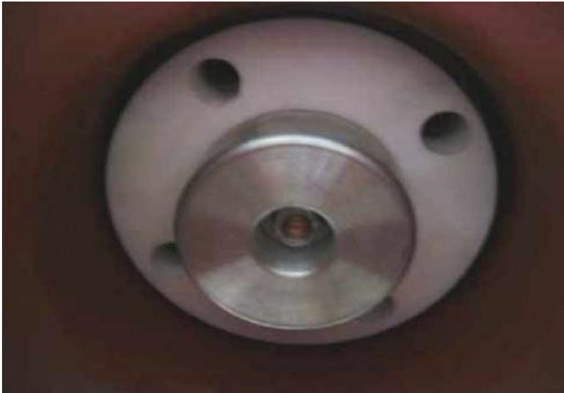
Figure 3.1: Internal UHF PD sensor mounted inside experimental 220 kV GIS system [78].
