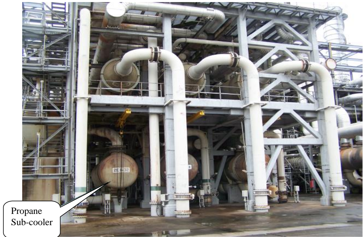
Figure 1.2: Picture of Propane Condenser and Sub-cooler at NLNG Plant
