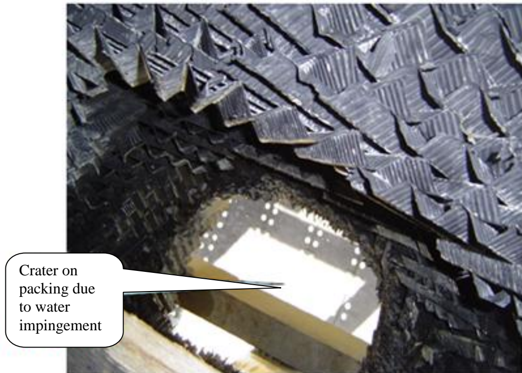
Figure 1.1: Picture of Damaged Packing of NLNG Cooling Tower
