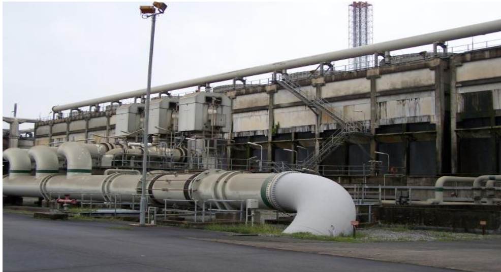
Figure 2.7: Picture of NLNG Plant Cooling Tower (9 cells)
