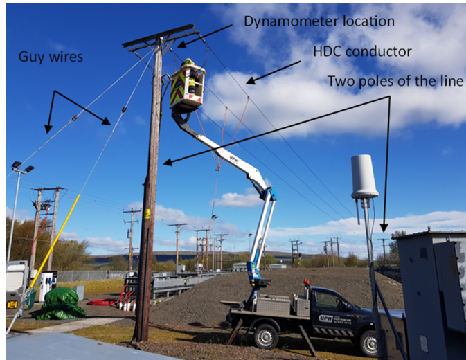
Figure 4.2: Overhead line at PNDC.
