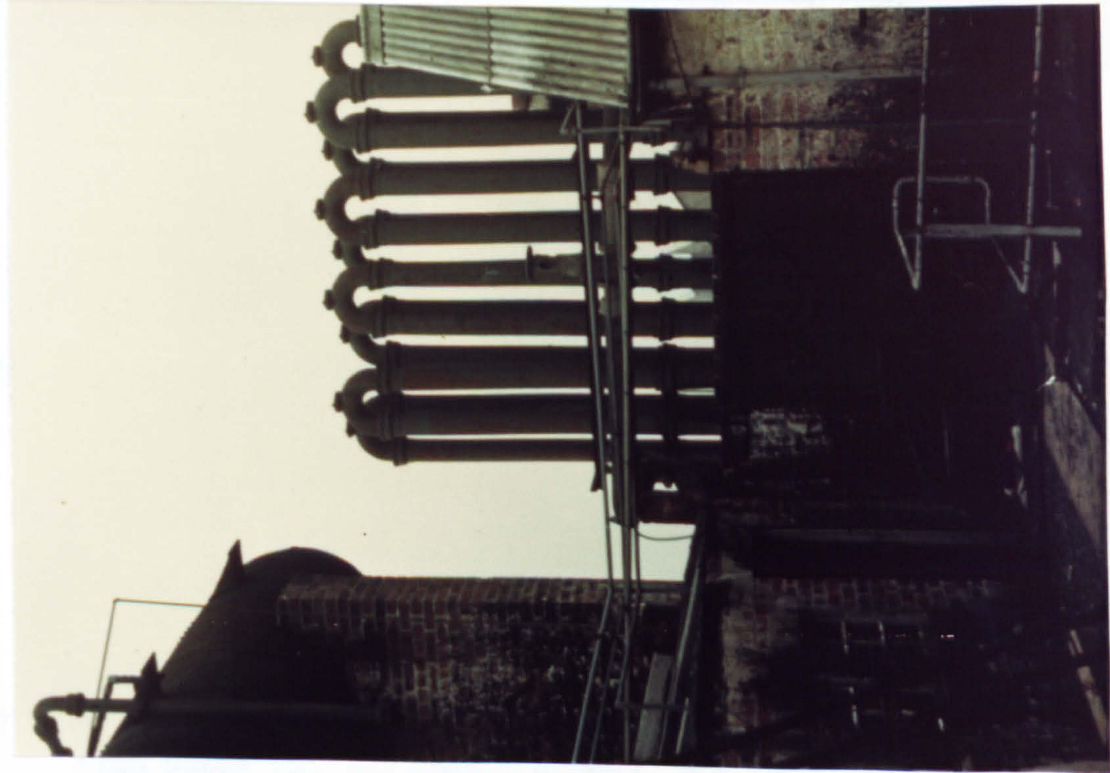
Fig 3.6 Condensers at Stranraer (1974) and Kirkconnel (1973)
