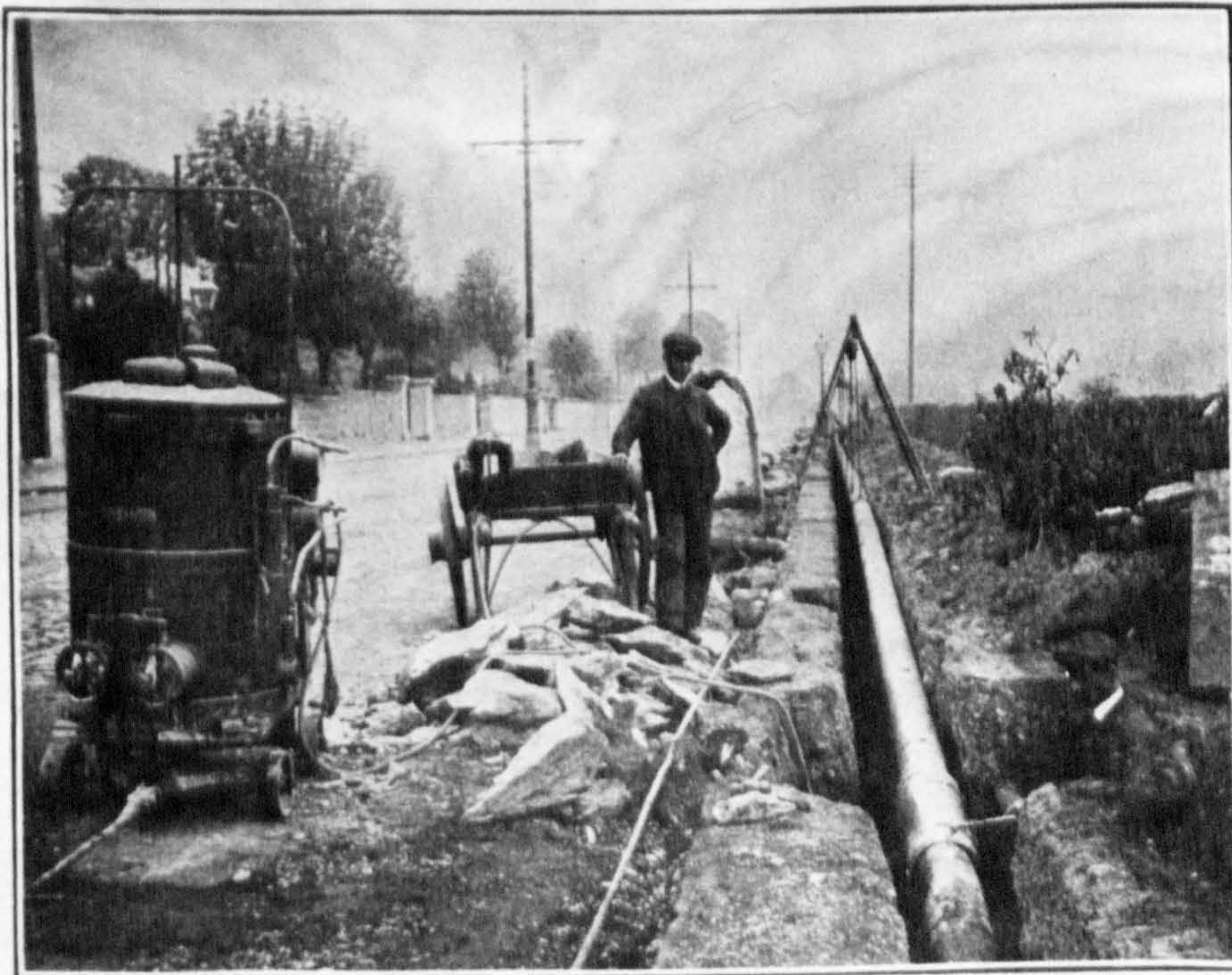
Steel Main, showing Hinged Cover to prevent melted bitumen falling on workmen when welding underneath.
