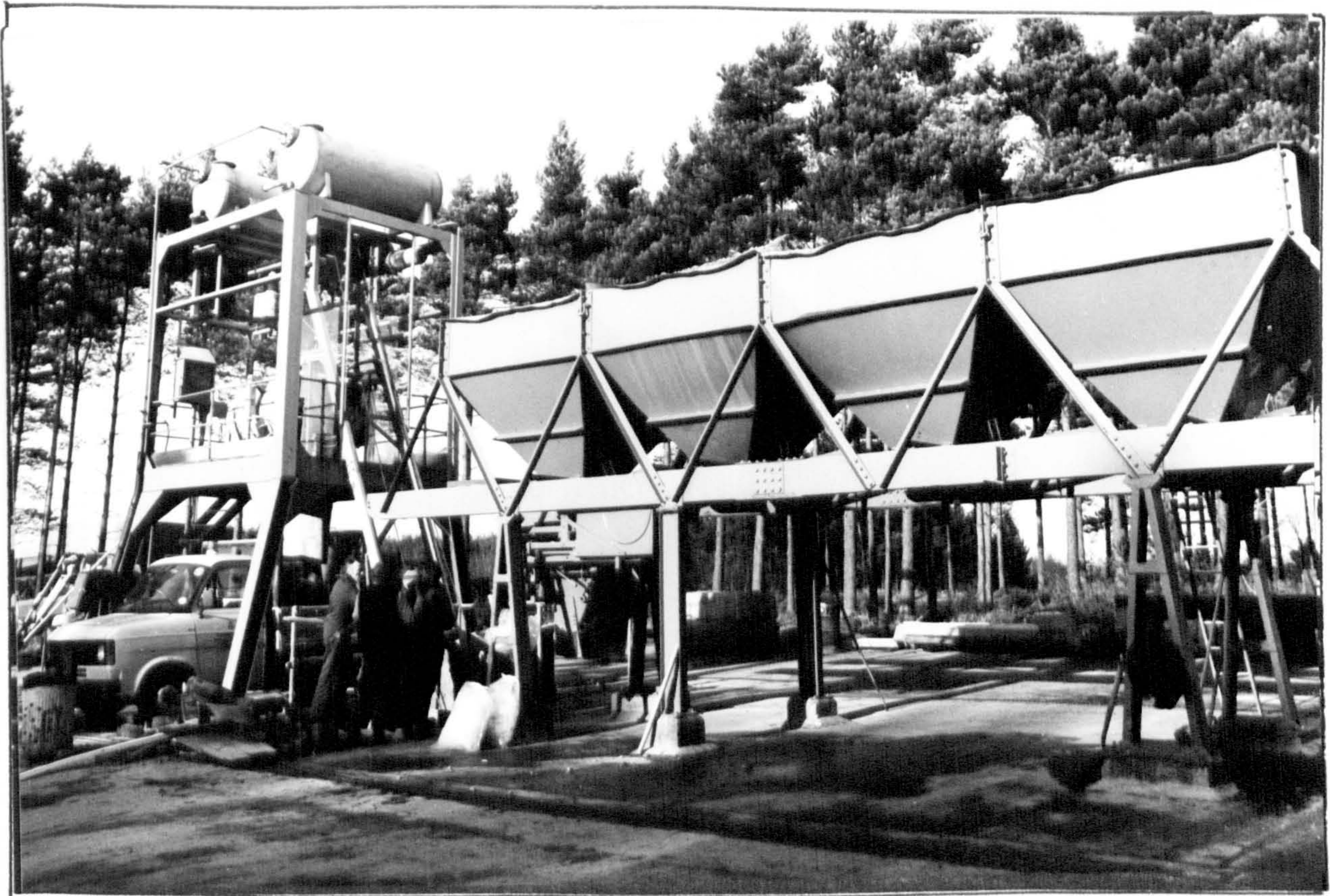
PLATE E.1 A View of the Batching and Mixing Plant
