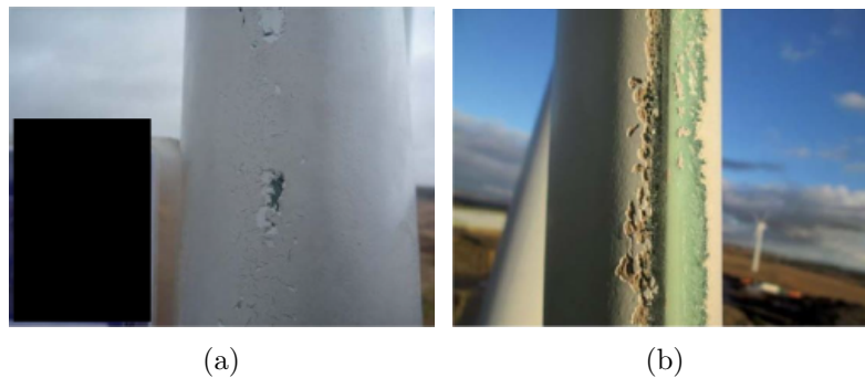
Figure 5.1: Minor (a) and major (b) erosion damage on the leading-edge of wind turbine blades (reprinted from [12]).
