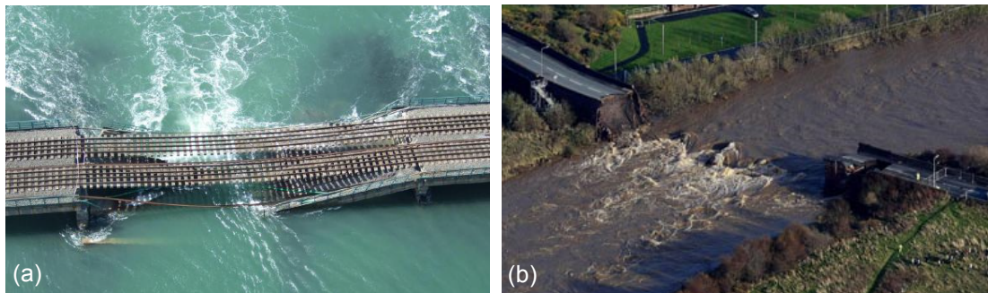
Figure 2.1: (a) The collapsed Pier 4 of Malahide viaduct (Ireland), source: RAIU, (2010). (b) The Northside bridge in Workington (Cumbria) during the floods in 2009, source: Byrne, (2009).
