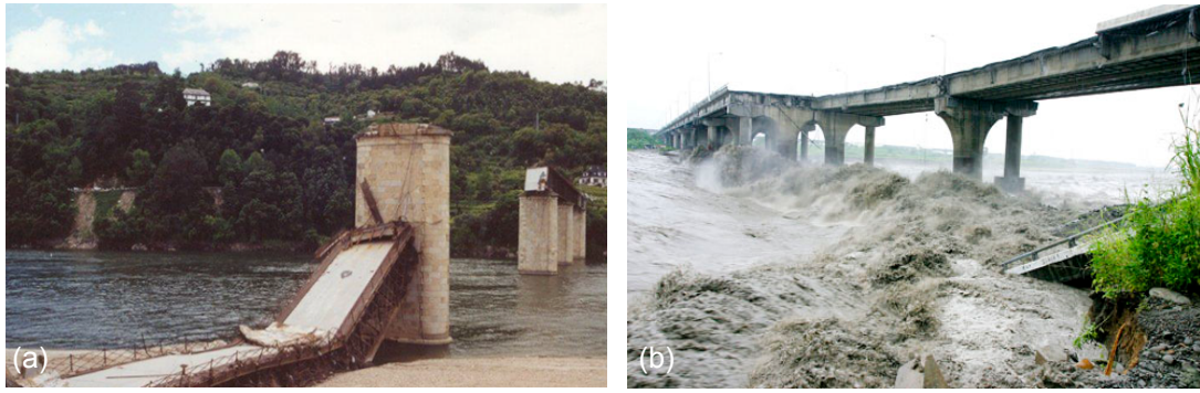
Figure 2.2: (a) Hintze Ribeiro Bridge failure (Portugal) due to scour of a masonry bridge pier, source: Briaud, (2011). (b) The collapsed Houfeng Bridge in Central Twain, source: Chao-Yang, (2008).
