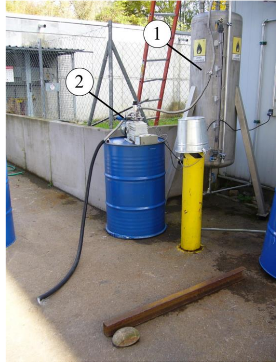
Figure 9.2: condensate reservoir of vacuum system, membrane pump
