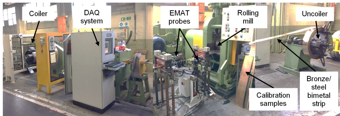
Figure 8.3: Industrial strip processing line with installed prototype EMAT inspection system
