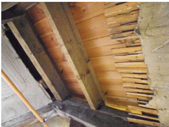
Figure 269: Recently replaced purlins and sarking boards in the roof of the North-West wing of Newhailes House
