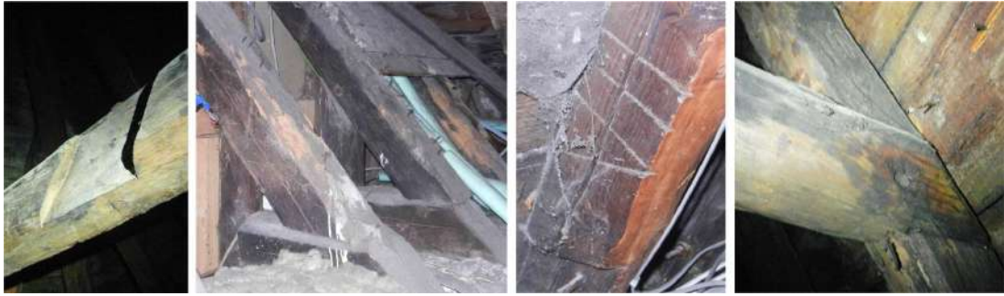
Figure 246: The roof of Cockenzie House: redundant joint on a collar (left), rafter feet (centre left), big sawn roman numerals on a rafter (centre right), lap joint between collar and rafter secured by metal nail (right)
