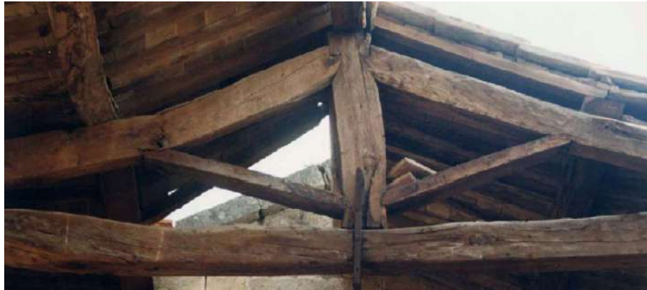
Figure 14: Failure of a rafter caused by the instability of the strut and favoured by a knot in the rafter and the notch for the joint; the efficient connection of the rafter to the post is the cause of the bending of the post (Tampone, 2007)
