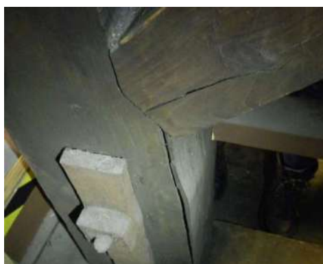
Figure 232: The roof of St Andrew and St George's church: compression cracks in a strut and in the joggle of a post
