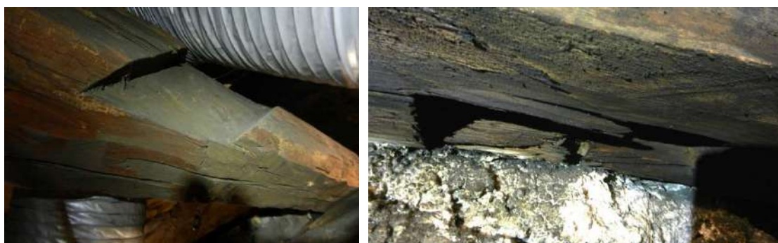
Figure 259: Redundant joints in purlin on West side of the roof of the North range of Holyrood Palace
