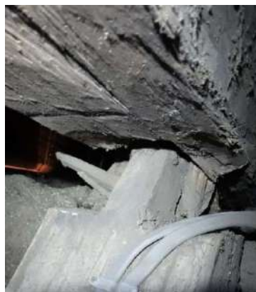
Figure 280: A failed joint between rafter and lower collar with an opening of 8cm in the roof of the long gallery at Pinkie House; the peg is broken
