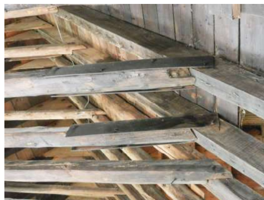
Figure 320: Repairs carried out in the roof of Methven Castle: many original rafters substituted with reused nineteenth century timbers, but many original collars retained and steel plates used to reinforce the lap joints between them
