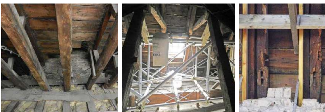
Figure 337: Past interventions: steel beam and ties counteracting the collars' deflection in Gardyne's Land (1675) (left), steel truss supporting the roof of Geilston House (1666) (centre), eighteenth century and twenty-first century timbers strengthening the original seventeenth-century timbers in Panmure House (1680s) (right)
