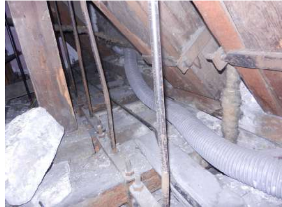
Figure 257: Strengthening of the rafter ends and floor beams on the South side of the North range of Holyrood Palace
