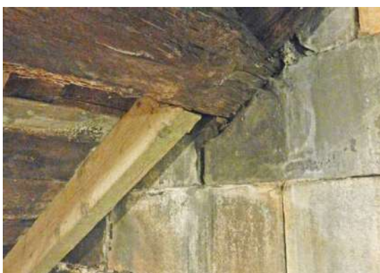
Figure 238: Fungi attack in the North-West gable of the roof of St Andrew's in the square church, affecting the butt-purlin, the common rafter and the sarking
