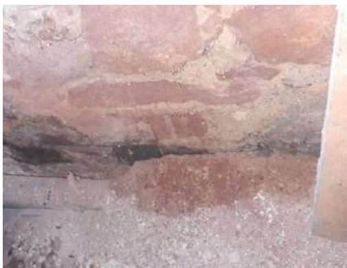
Figure 305: The dampness disintegrating the East gable in the roof of the North range of Touch House
