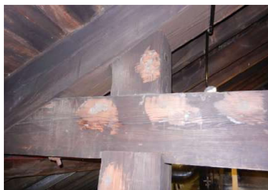
Figure 239: Resin injections used in 1980s to treat insect attack in the roof of St Andrew's in the square church
