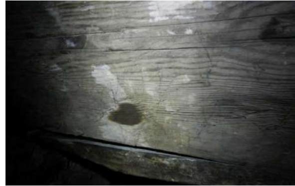
Figure 308: Fungi attack on a purlin of the roof of the central block of Touch House, near a gable wall
