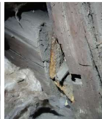
Figure 281: A failed joint between rafter and lower collar with an opening of 4cm in the roof of the long gallery at Pinkie House; the rafter is broken
