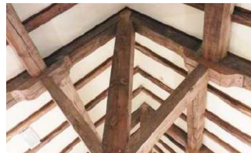
Figure 167: Cleats used to reinforce the joint between struts and rafters in the trussed roof of Brodie Castle Stables (end eighteenth century)
