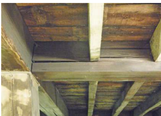
Figure 240: Cracks in a butt-purlin of the roof of St Andrew's in the square church
