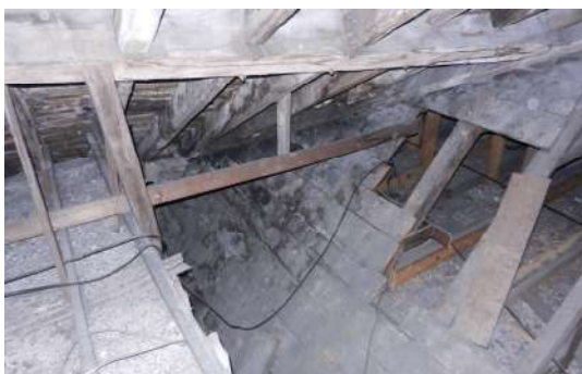
Figure 303: Remains of sarking on the North side of the roof of the North-West range of Touch House
