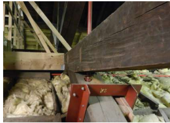
Figure 243: A joint between strut and collar with steel strengthening interventions added in 1990s in the roof of St Andrew's in the square church
