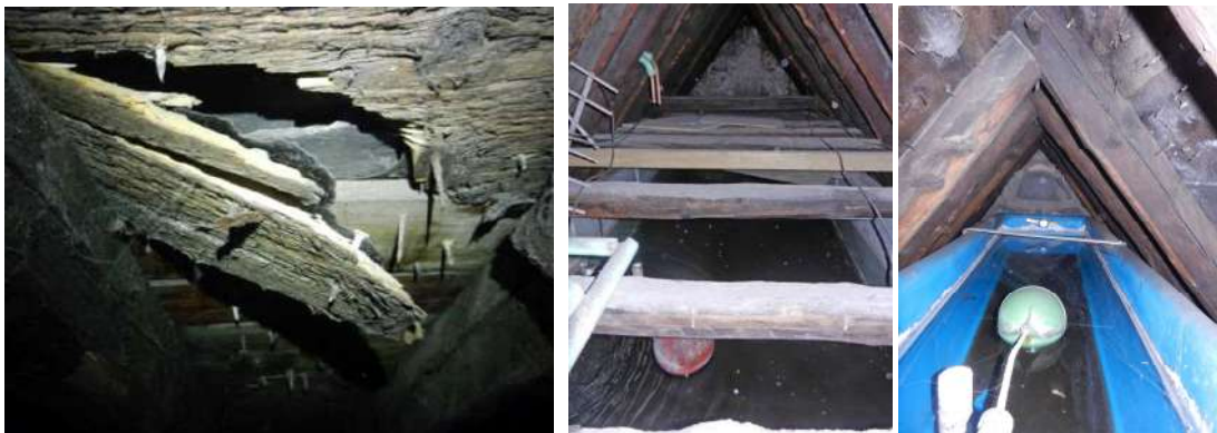
Figure 248: Broken sarking in the roof of Cockenzie House
