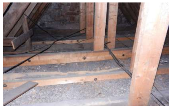
Figure 304: Additional collars and struts reinforcing the roof of the North-West range of Touch House
