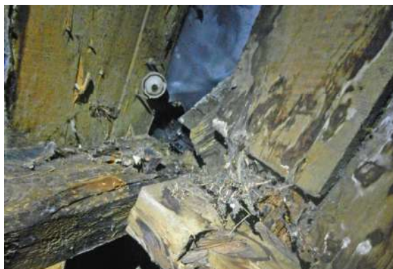
Figure 306: Broken sarking in the roof of the North-West range of Touch House
