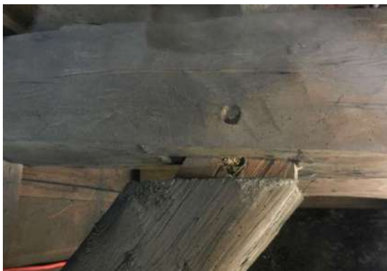
Figure 262: A degraded peg causing the disconnection and slip of a joint between rafter and upper beam of the roof of the North range of Holyrood Palace
