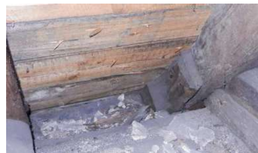
Figure 169: Cleats used to reinforce the connection between rafters and purlins in the common rafter roof of Touch House (end seventeenth century, but the purlins might be a later addition)
