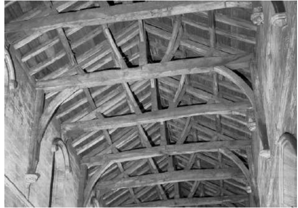
Figure 110: The roof of the central nave of Holy Rude church in Stirling (1455) (RCAHMS SC 738897, 1959)
