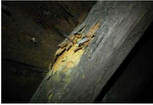
Figure 252: Insect attack on a rafter in the roof of Cockenzie House
