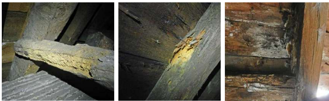
Figure 331: Material degradation in common rafter roofs: old insect attack in Mallyen House (1635) (left), active insect attack in Cockenzie House (1680s) (centre), fungi attack in Kelburn Castle (1581) (right)
