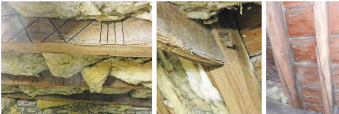
Figure 285: The roof of the King's Old Buildings: tool and carpentry marks on collars (left), mortice and tenon joint between rafter and upper collar (centre), scarf joints in rafters (right)
