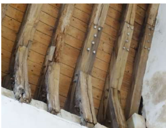
Figure 319: Repairs carried out in the roof of Alloa tower: some rafter ends, sole pieces and ashlar posts partly replaced with new timber and connected to the original timber with scarf joints and steel bolts
