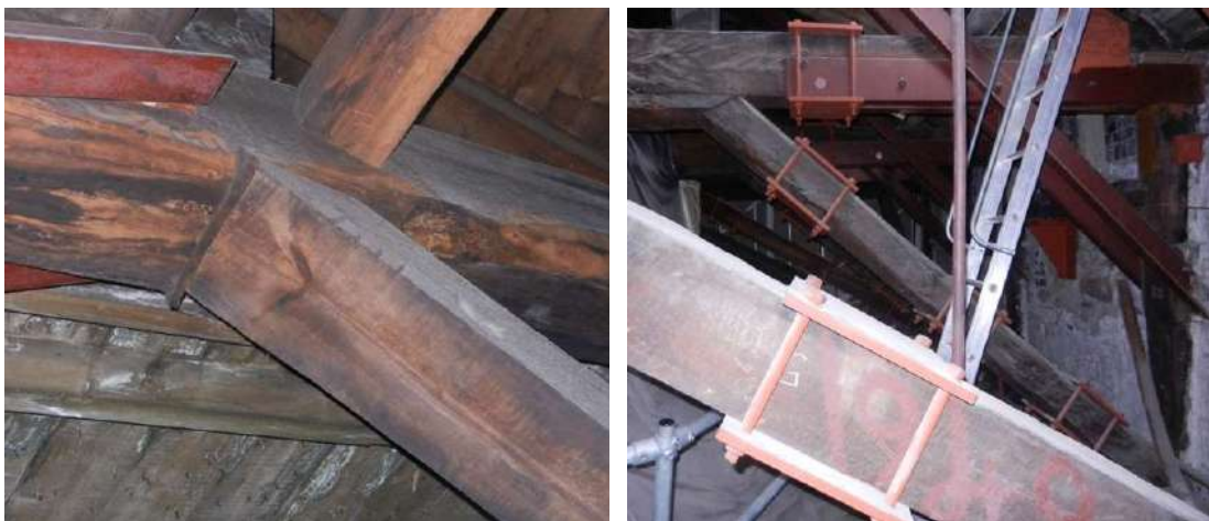
Figure 222: Repair works to the roof structure of Glasgow Trades Hall (1791-4): a timber wedge inserted between a slanted brace and a horizontal beam (left); steel rods, plates and brackets added in 1990s (right)
