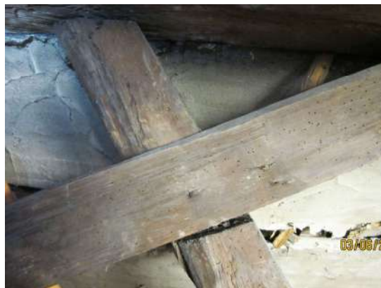
Figure 270: Cross joint between struts with an opening of 1cm in the roof of the North-West wing of Newhailes House
