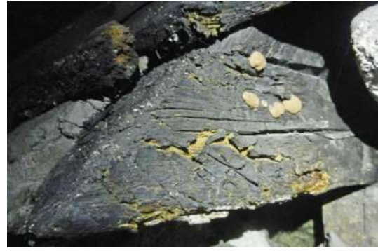
Figure 253: Fungi attack on a rafter foot in the roof of Cockenzie House
