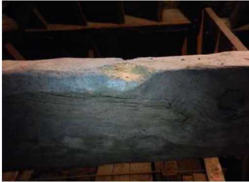
Figure 307: Insect attack on the West side strut of the roof of the central block of Touch House
