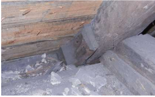
Figure 301: A cleat reinforcing the joint between a rafter and a butt-purlin in the roof of the North-West range of Touch House
