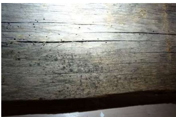
Figure 292: Fungi attack on a purlin in the North-West corner of Stirling Castle Palace
