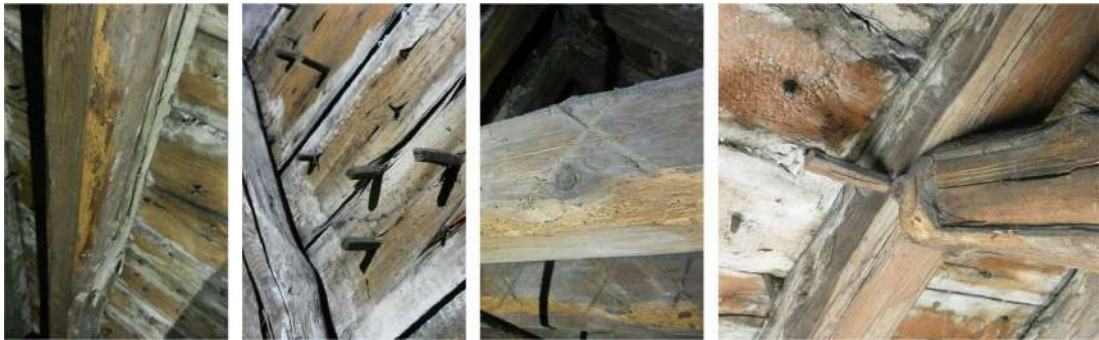
Figure 274: The roof of the long gallery at Pinkie House: the dressing of the rafters (left), the oak pegs securing the slates to the sarking (centre left), carpentry marks on collars (centre right), mortice and tenon joint between rafter and collar secured with a timber peg (right)
