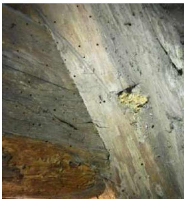
Figure 279: A degraded peg in a mortice and tenon joint between rafter and upper collar in the roof of the long gallery at Pinkie House
