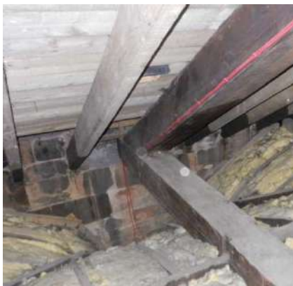
Figure 177: Connection with the wall in St Andrew's in the Square church (1751-3): the tie-beam simply sits on the ashlar masonry
