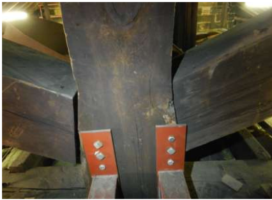
Figure 242: Rotation of the central post causing the opening of the joint with the strut and steel strengthening interventions added in 1990s in the roof of St Andrew's in the square church
