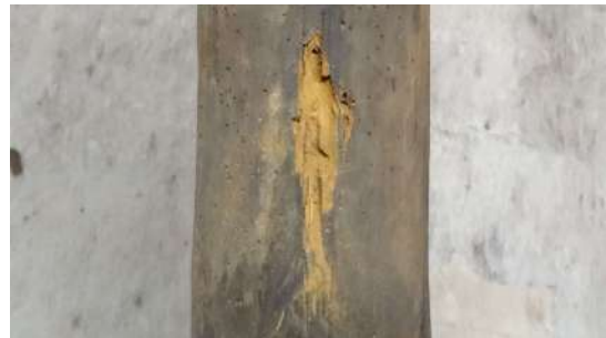
Figure 261: New bore dust suggesting active attack on a strut of the roof of the North range of Holyrood Palace
