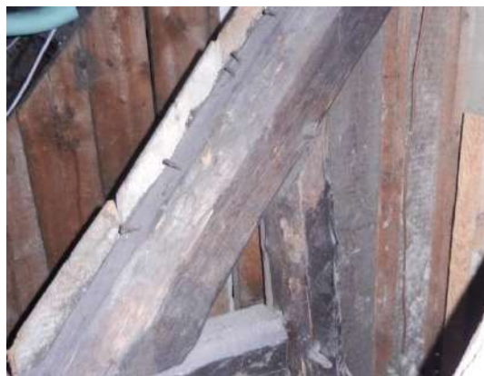
Figure 181: Nails on rafter feet of Cockenzie House (1680-3) left after the removal of the sarking boards
