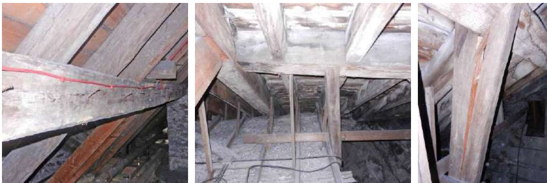
Figure 329: Mechanical damage in purlin roofs and complex frames: deflected purlin in Melville House (1697-1701) (left), deflected purlin in Touch House (1757-62) (centre), crack in strut supporting the purlin in Touch House (1757-62) (right) (Serafini and Gonzalez Longo, 2016)
