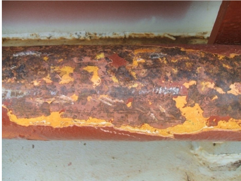
Figure4.17. An example of bad surface cleaning done by hammer
