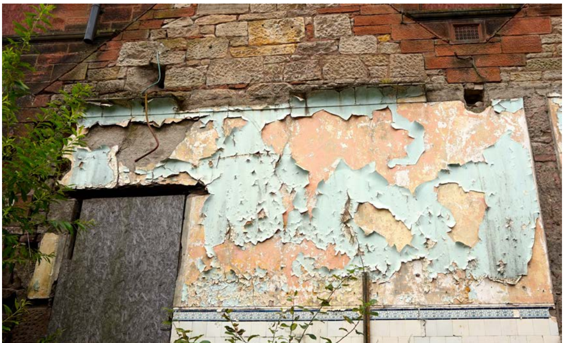
Figure 6.14: ‘Peeling paint’, Author’s own photograph
