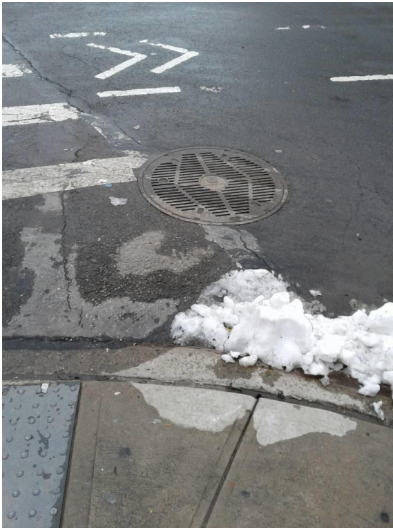
Figure 15. A photograph of a drain basin obtained by Matthew
